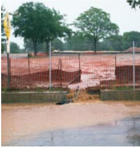
Figure 6. Construction site with inadequate sedimentation 95
